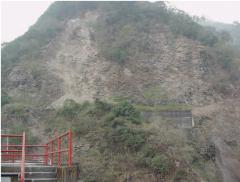
Figure 12. Picture showing the local slumping occurring on the wall off the slope in the Wushieh Reservoir, Taiwan, from the 921 Chi-Chi Earthquakes.
