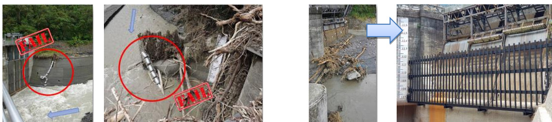
Abb. 16: The failed debris booms in barrages. Abb. 17: Water intake barriers of Guishan Dam.
