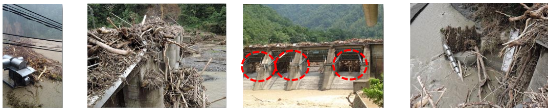
Abb. 8: Serious damage caused by woody debris.
